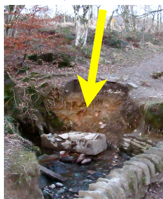
Foundation of old bridge now collapsed into stream.
